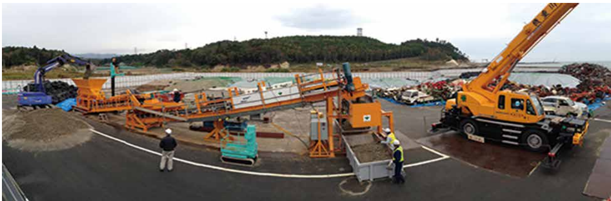
Amec Foster Wheeler's ScanSort system at work in Japan
