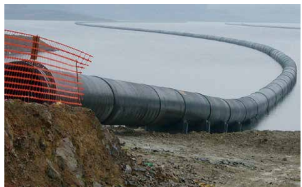
Seawater intake pipe
