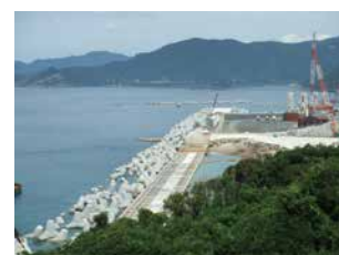
Shimane nuclear power station
